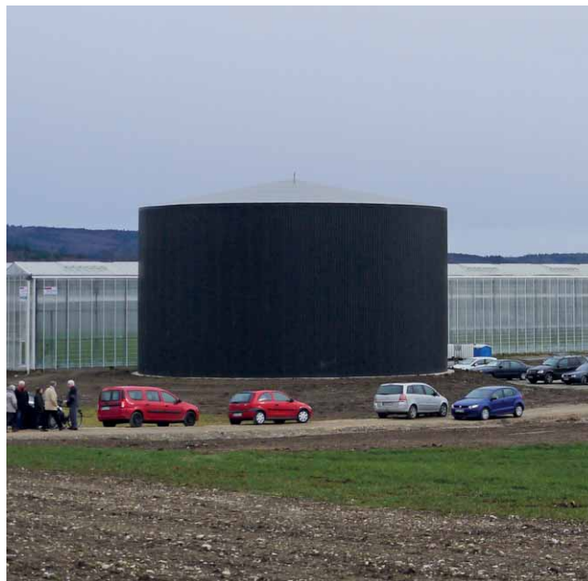
Newly built heat storage tank for the greenhouse in Aach.
